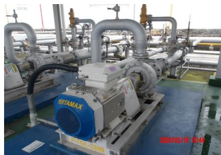
Figure 1. MCPK 125-100-400 CC centrifugal pump and its technical specifications used in the Pertamina fuel distribution system at PT Pertamina Patra Niaga Fuel Terminal Tegal. B. Pump Capacity Analysis
