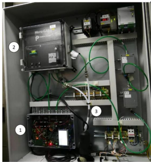
Figure 2. Internal components of a switch cabinet installed on a container ship
